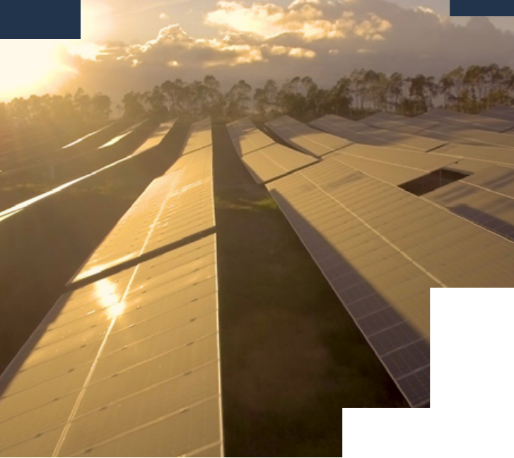
Solar farm at Summerhill Waste Management Centre
